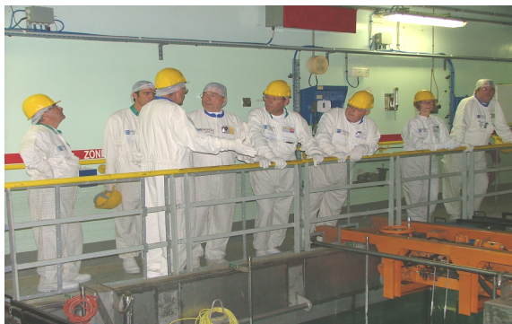
Cooling Pool at the CPEN in Gravelines, 10 May 2007
